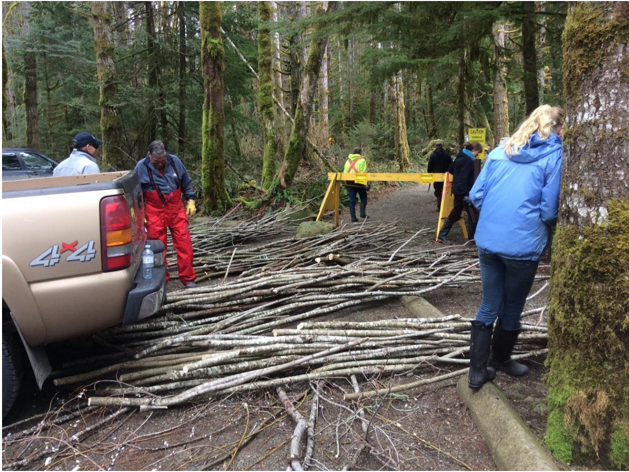
Unloading live willow stakes for riparian restoration work in Rosewall Creek parking lot area. Live stakes were sharpened (using an axe) so that they could be driven into the ground more easily.
